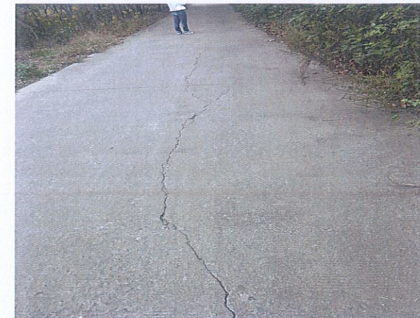
K0+275~K0+290 处连续纵向裂缝
